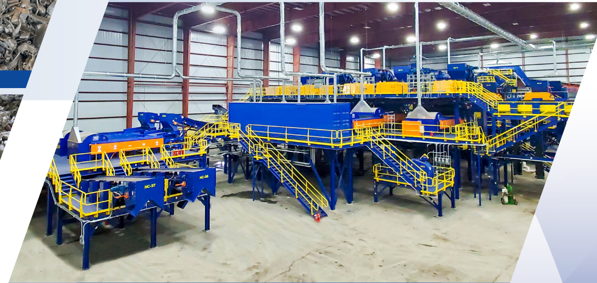
70 TPH Non-Ferrous Recovery Plant
